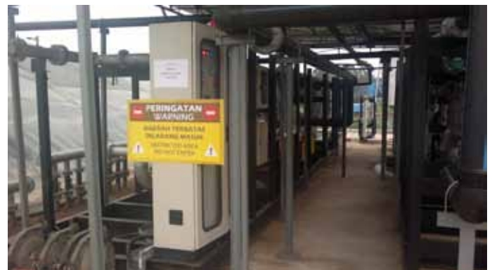
Biogas from palm oil mills effluent (POME) in PTPN V, Riau. (Source: EEP Indonesia)
